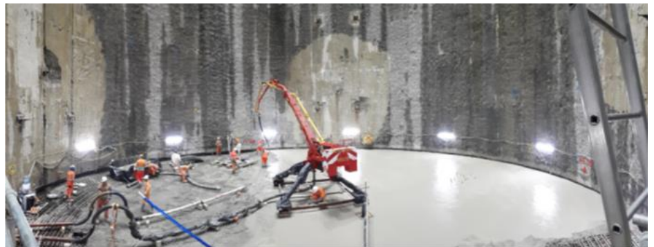
This photo was taken whilst pouring the base slab at our Chambers Wharf site in Bermondsey
