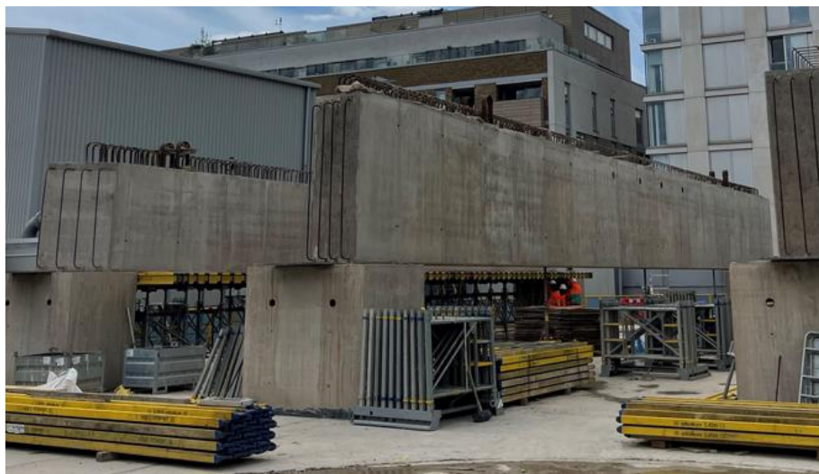
Image shows the concrete beams which will be moved into the acoustic enclosure to eventually form part of the permanent shaft roof slab
