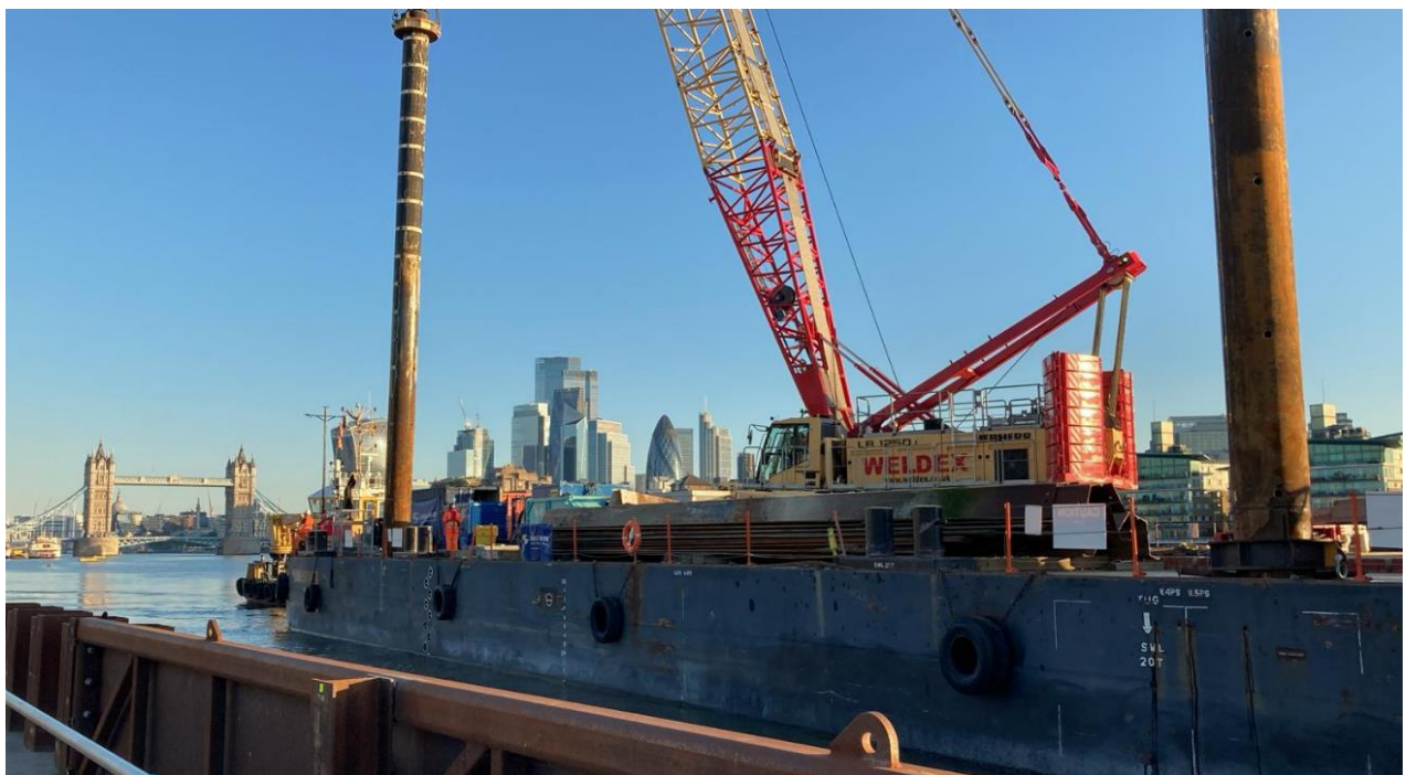
This picture shows the barge delivery of sheet piles from the Tideway King Edward Memorial Park site, which will be re-used at Chambers Wharf
