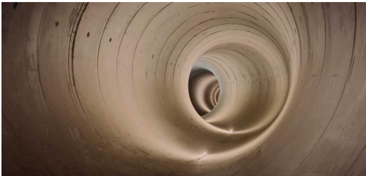
A section of the tunnel in west London (the lights have now been removed)
