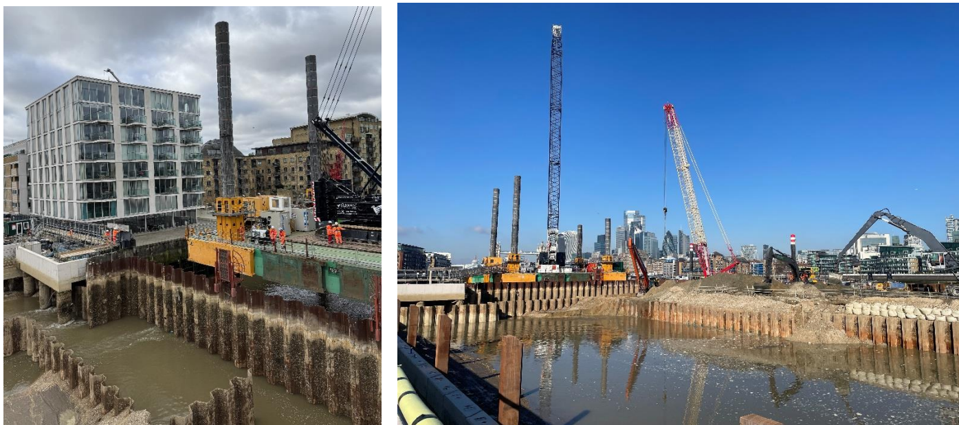
Photograph shows the jack-up barge at Luna House and from the river wall
