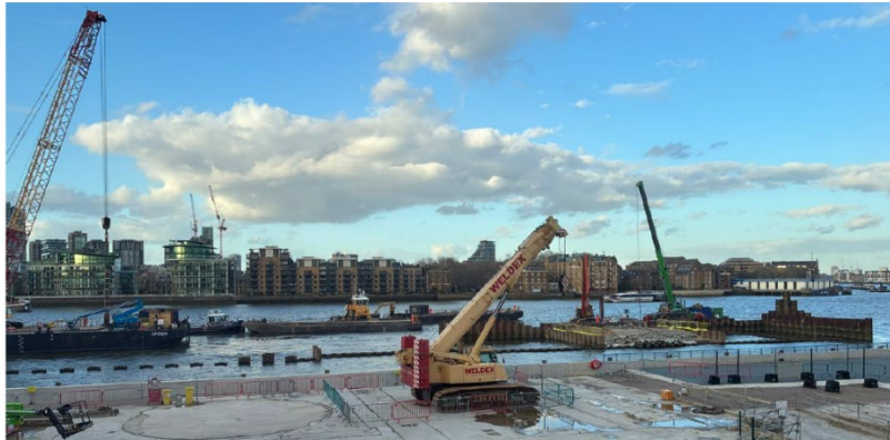
Image shows a view of cofferdam island excavation downstream (R) and sheet pile extraction upstream (L)
